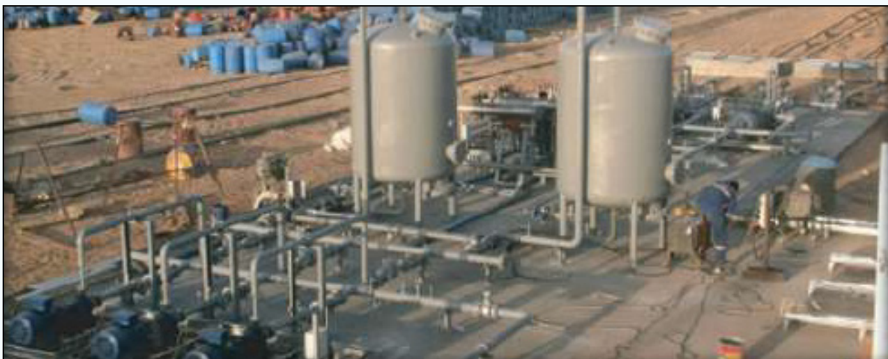
WATER FILTRATION & PUMPS AREA–DAPETCO
