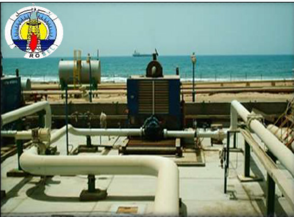
WATER INJECTION PUMPING STATION (AGIBA: MELIHA FIELD)
